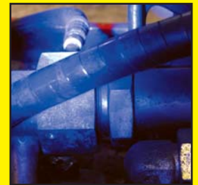
The site is then re-inspected with the lamp. No glow means that all leaks were repaired successfully.
