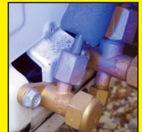
The site is then re-inspected with the lamp. No glow means that all leaks were repaired successfully
