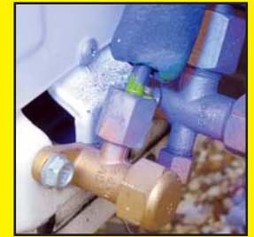
Every leak will fluoresce a brilliant yellow-green pinpointing the exact source of every leak
